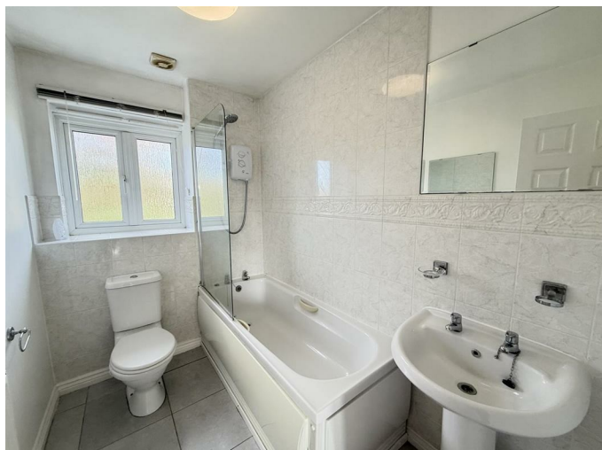
Fitted with a white low flush WC, pedestal wash hand basin and panelled bath with electric shower system over, tiled surrounds, extractor fan, opaque window to rear aspect.
